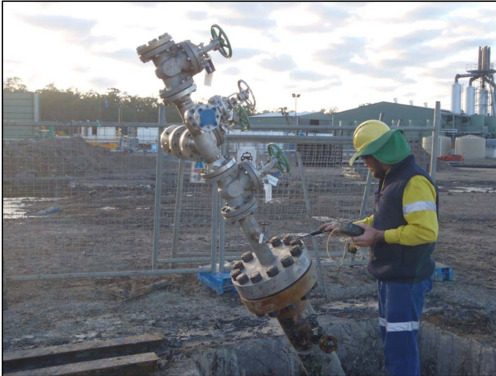
Panel 2 - injection well head
